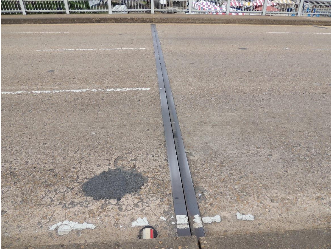
Condition Photo 2: Open joint at bent 3 locked in the closed position and a patched concrete deck spill.
