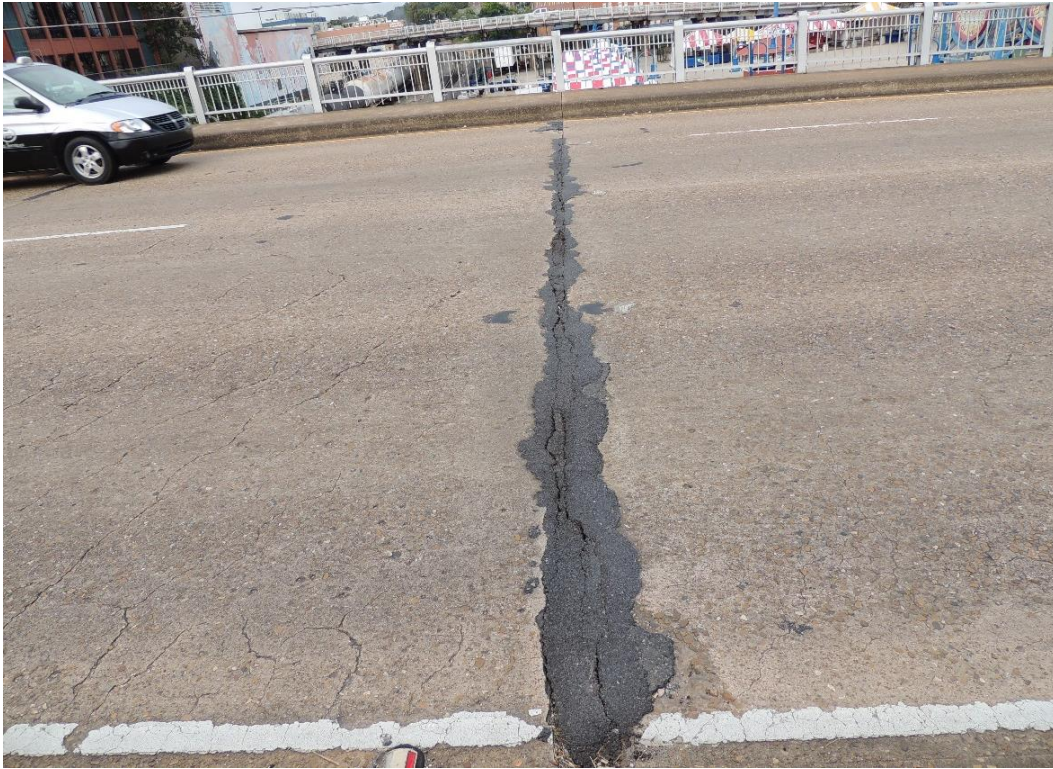
Condition Photo 4: Asphalt patched pour seal deck joint at bent 4, as well as transverse cracks and exposed aggregate and wear.
