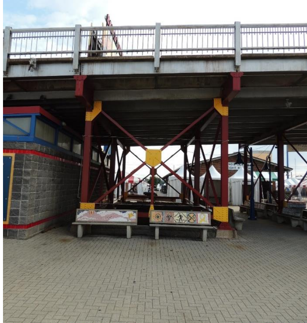
Character-defining Feature Photo 2: Design and construction of a railroad grade-separation overpass. The steel I-beam spans, which crosses the railroad, and adjacent concrete deck girder spans comprise the superstructure. Detail of span 2.
