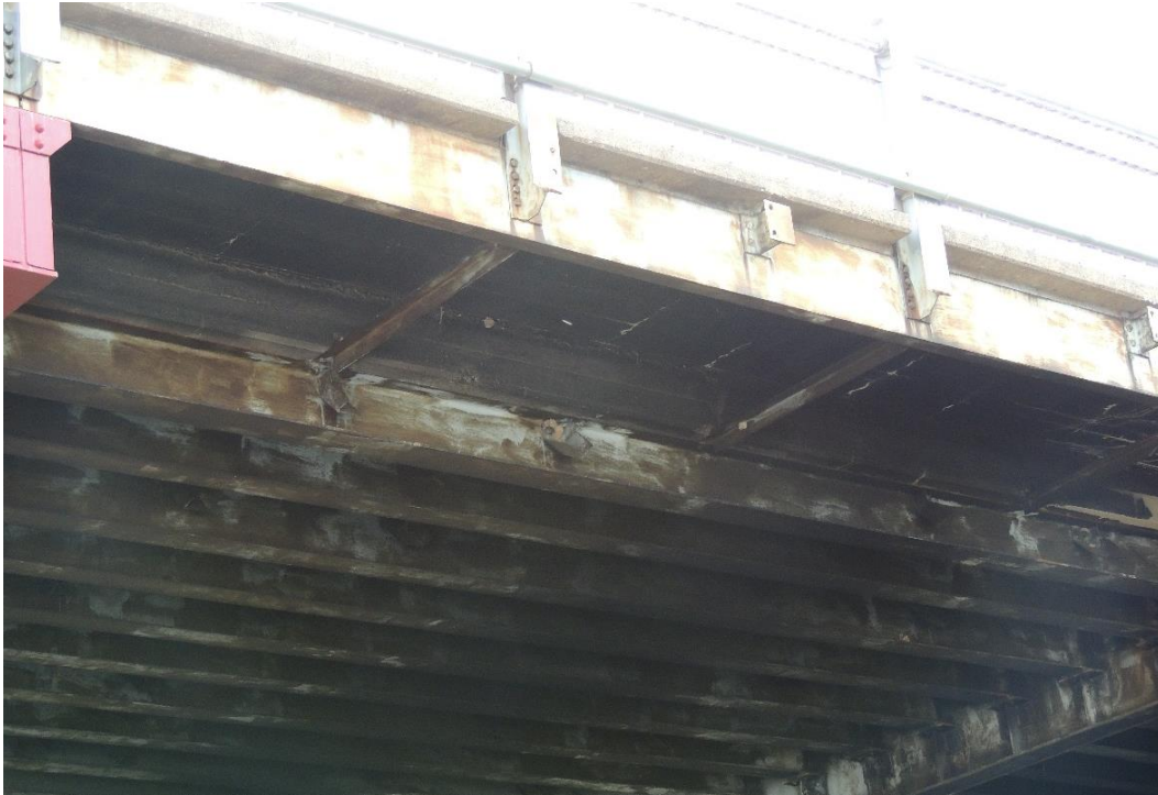
Condition Photo 8: Span 4 staining with soot from the locomotive exhaust.
