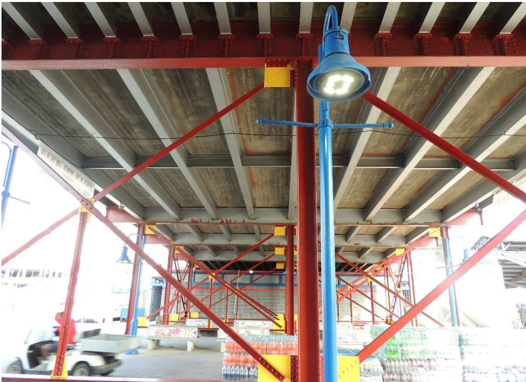
Condition Photo 11: Paint failure of the steel floor system and longitudinal cracking and efflorescence.
