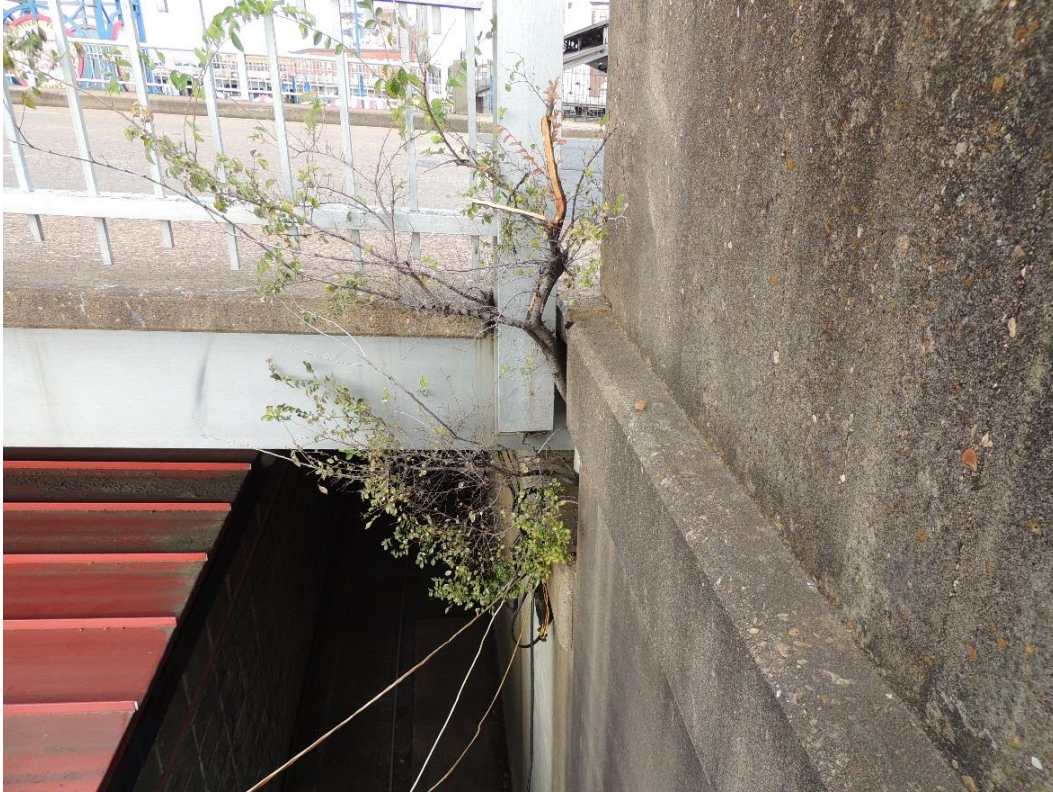
Condition Photo 6: Vegetation growth from the north abutment wall.
