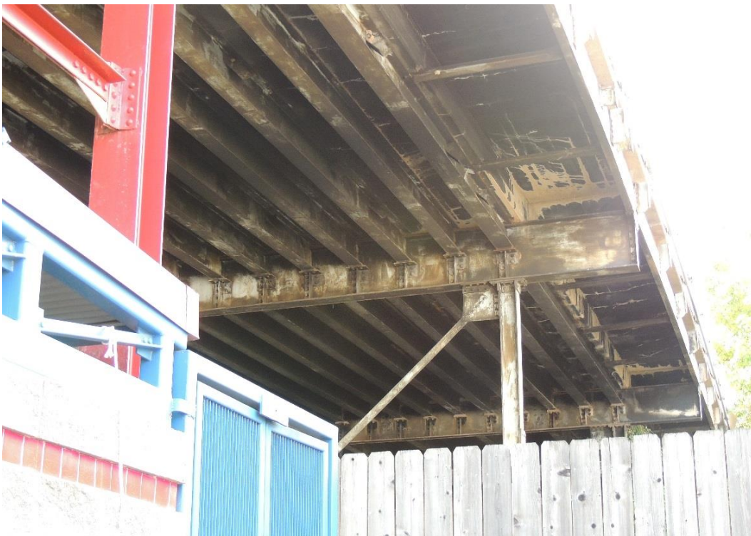
Condition Photo 9: Spans 3 and 4 stained with soot from the locomotive exhaust.
