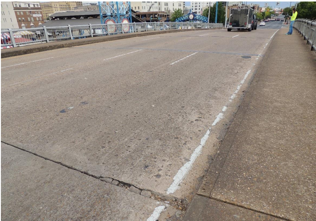
Condition Photo 3: Spalled concrete at pour seal deck joint at bent 2.
