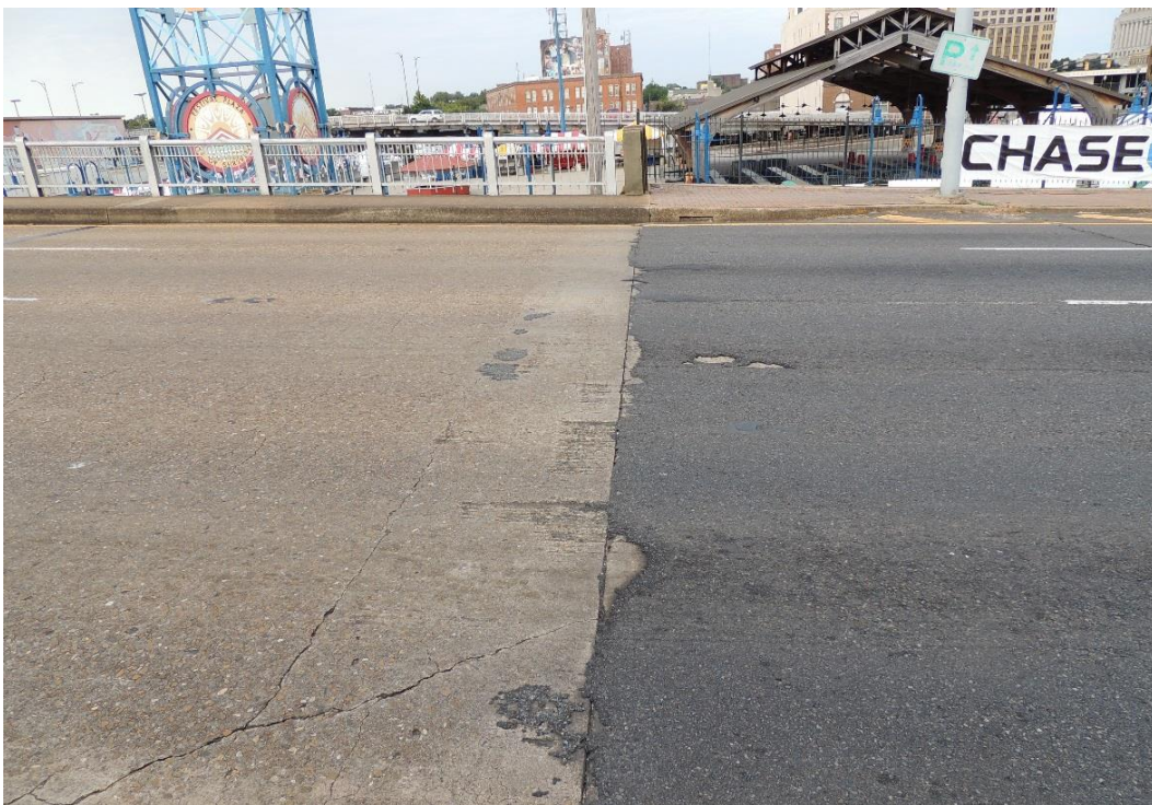
Condition Photo 5: Spalled concrete to asphalt transition at north abutment.
