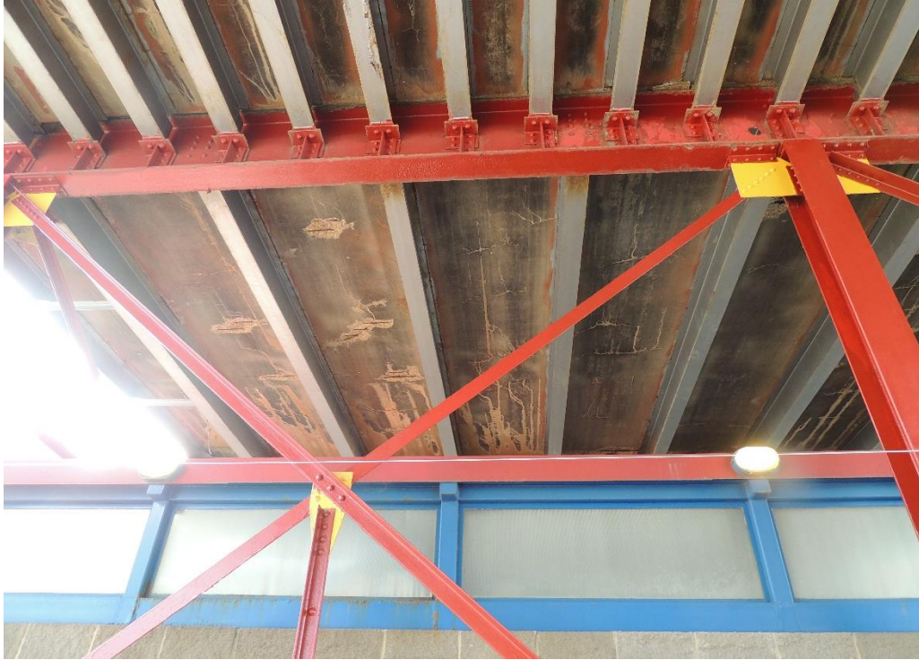
Condition Photo 10: Transverse deck cracking with efflorescence and exposed steel, as well as paint failure on the floor system.
